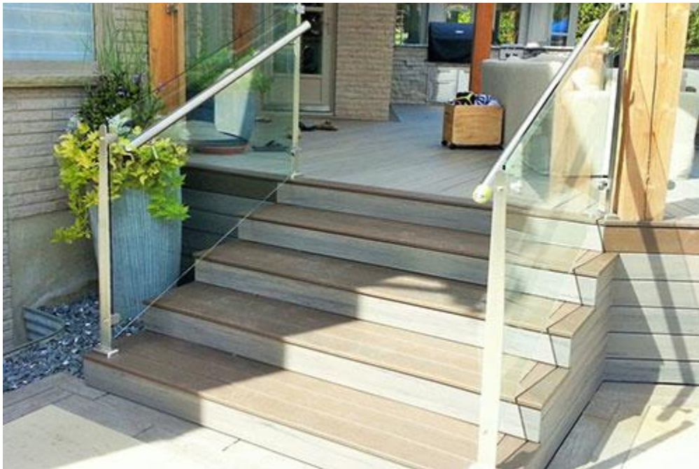
Glass mounted handrail brackets supporting SS handrail with domed ends.
