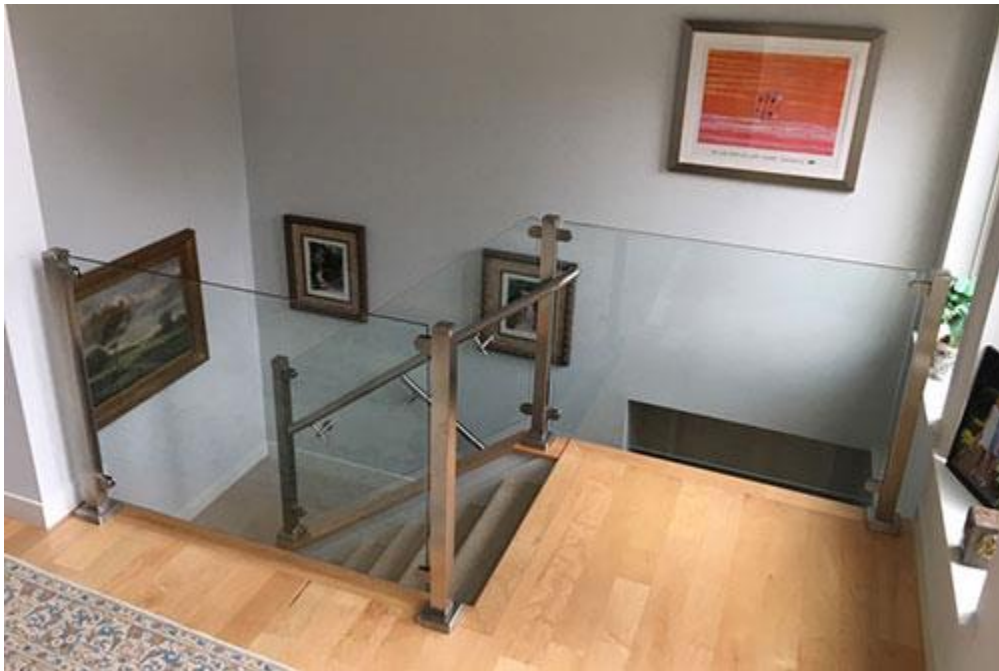
Glass mounted handrail brackets supporting SS handrail with end return fittings.
